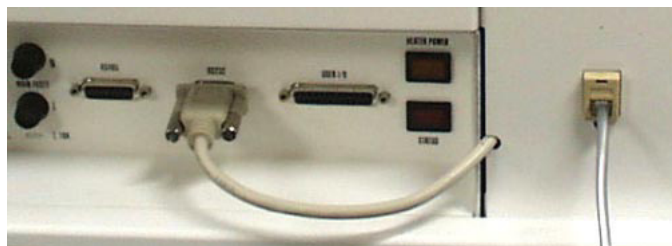
Detail of serial connection from Partisol-Plus Sampler to modem and RJ-11 jack to outside telephone line.
