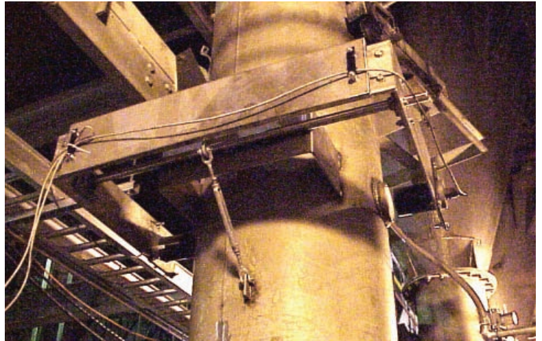
Shown above is a Ramsey Microwave Point Level Detector installed on a pressurized coal downspout with a custom mounting bracket.
