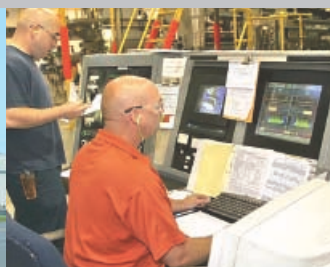
In the Control Room
